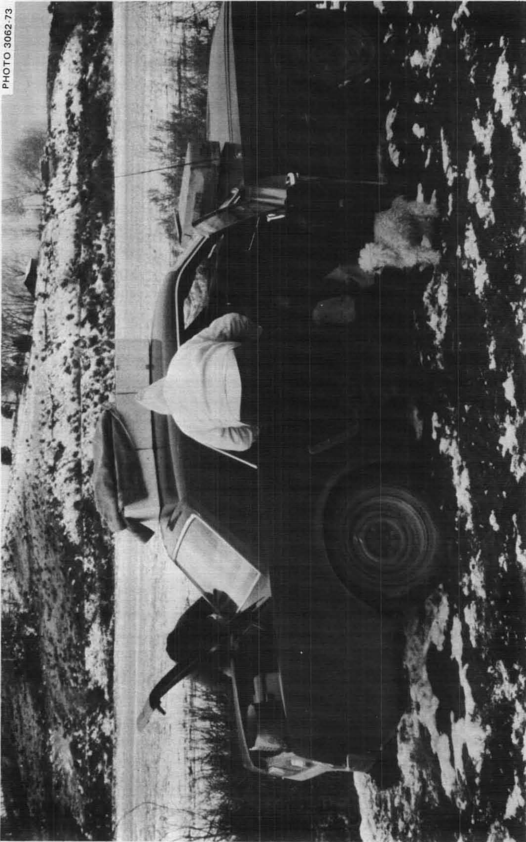
Fig. 6.5. Unloading tools, food, and water at the building site on the Kearny farm about 5 miles from Montrose. Work on the shelter began at 10:11 AM. This family brought along two items that were not on the Evacuation Check list (and will not be), but which they said they would carry with them in a real evacuation: their .38 automatic with extra ammunition and their toy poodle. Both the pampered poodle and daughter stayed in the car almost all of the time.
